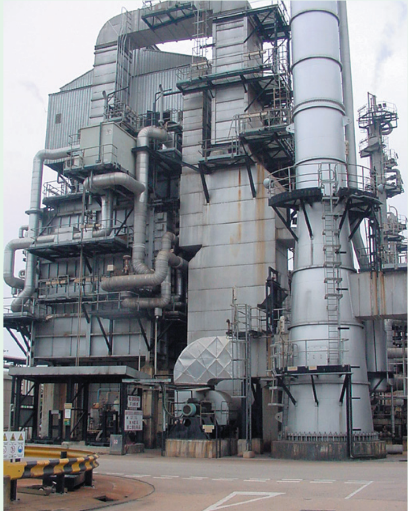
Hong Kong Gas Reformer Furnace ID Fan
